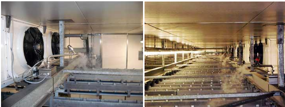
Figure 2. Germ elimination modules in front of circulating air cooling units (air-solution.com)
